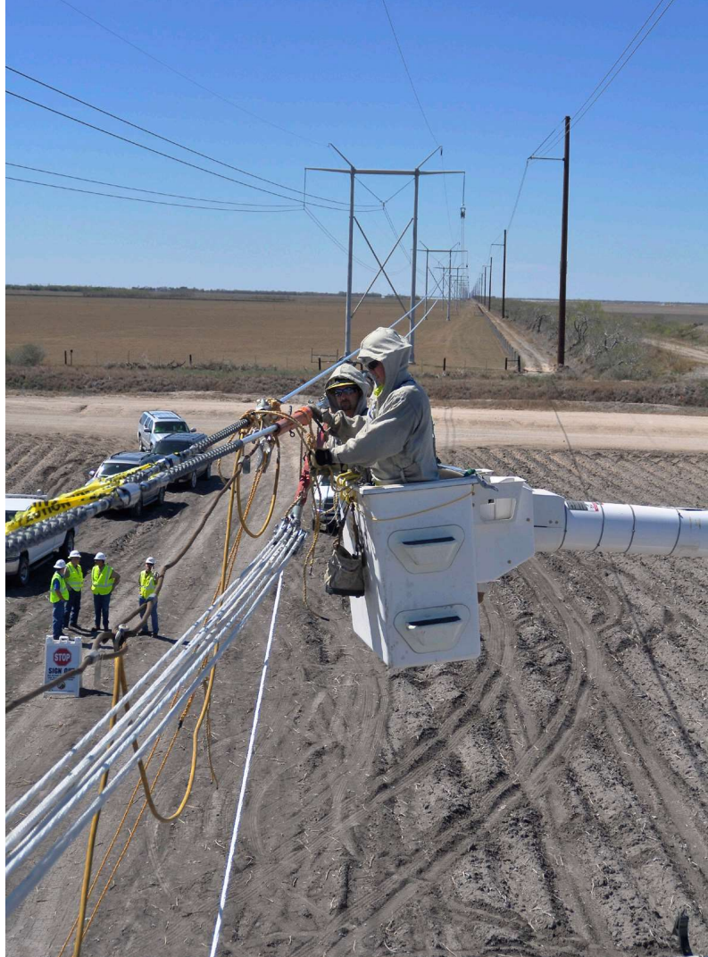
AEP 345 kV ACCC Reconductor Project
