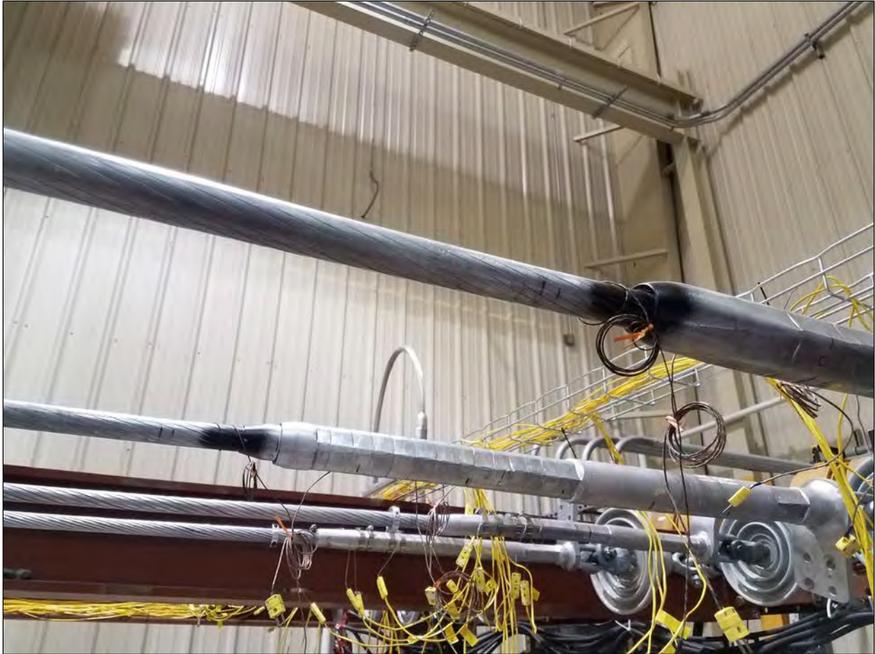
Figure 6-2 Burndy and AFL dead-ends (in the foreground) after 1500 cycles
