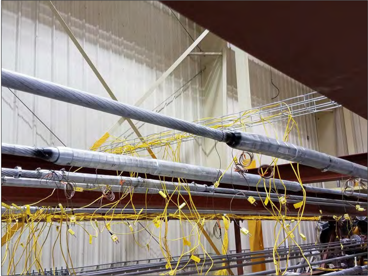
Figure 6-3 Burndy and AFL splices (in the foreground) after 1500 cycles
